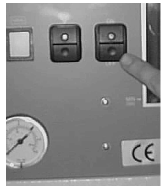
Switch ON right button (MAIN)
